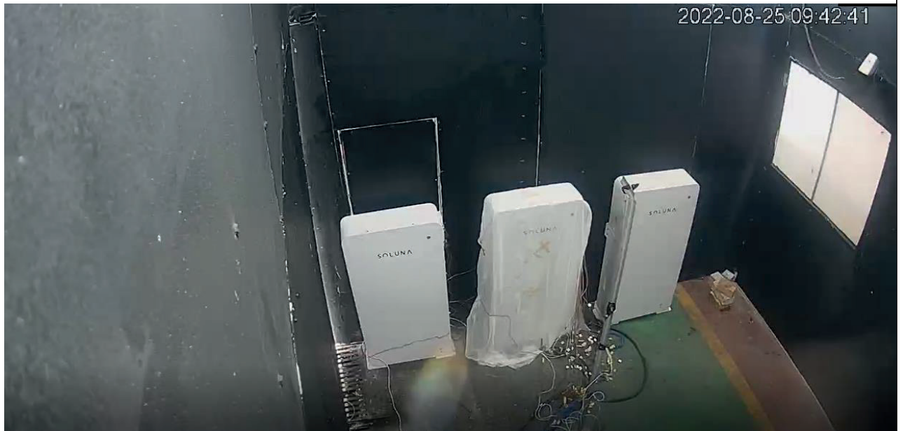
Unit during test
